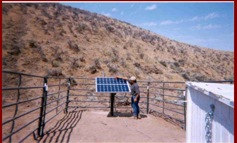
A Solar Panel was installed to power the solar pump which is housed in the insulated pump house fenced off from livestock.
