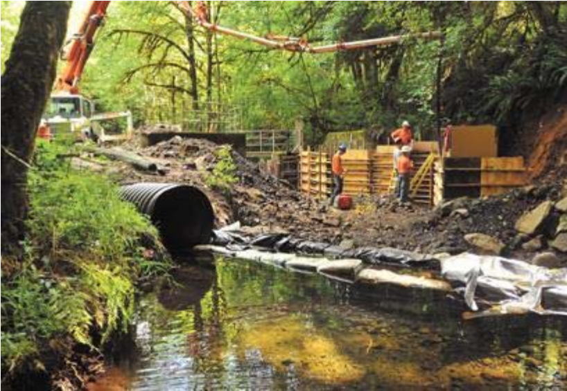
Casey Campbell/Gazette-Times Contractors pour concrete for a fish ladder around an intake dam on Griffith Creek, a tributary of Rock Creek west of Corvallis. The work is part of a $750,000 project to open the city's 2,400-acre Rock Creek Watershed to migrating cutthroat trout.
